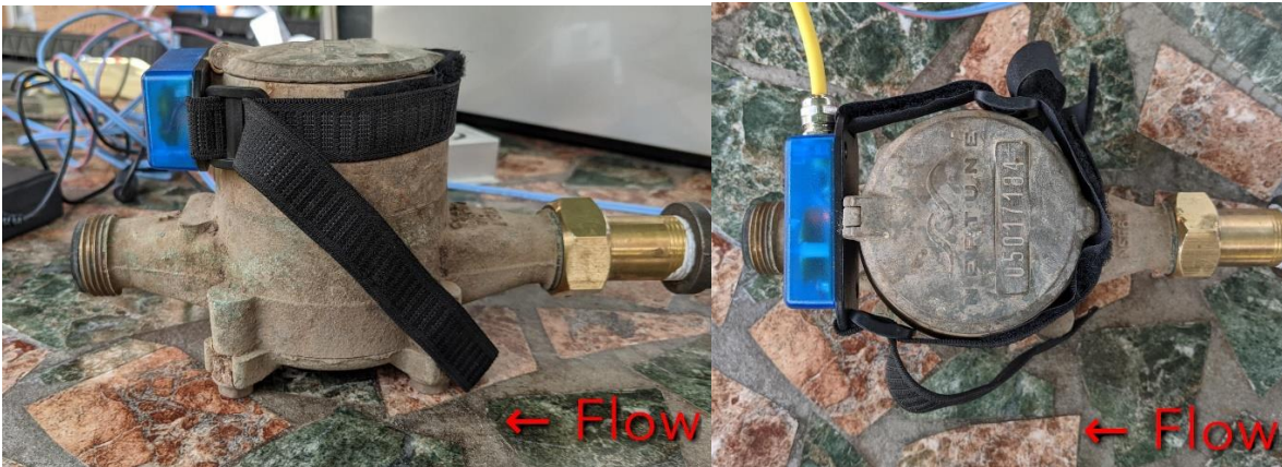
Logger placement on Neptune T-10 (side view) (overhead view)
